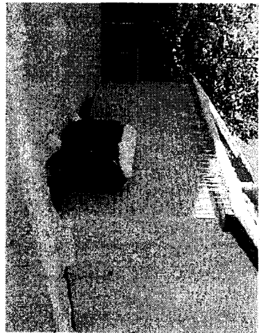
Lennox Island First Nation Furnace oil tank at "old" pumphouse.
