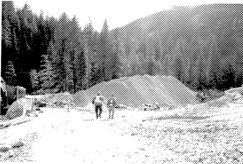
Figure 1. Construction at Stave intake site. Note pile of crushed rock in background (Stave river is ~ 20 m from the pile on the opposite side).
