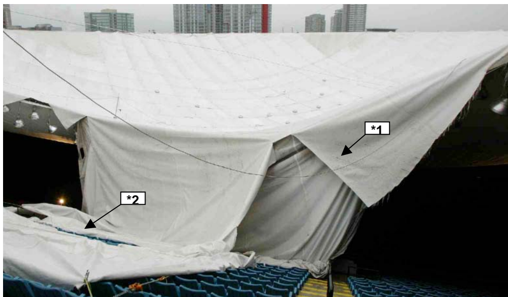
Figure A1-2: Damaged Triangle Panel, Jan 6, 2007.
